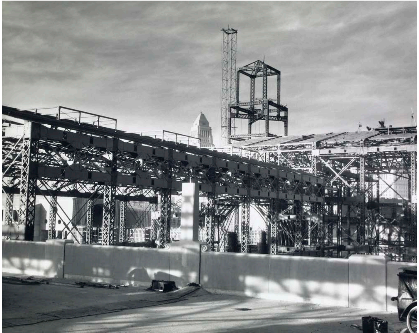
Construction of the Los Angeles Union Passenger Terminal, John and Donald Parkinson, photographed in 1933.
