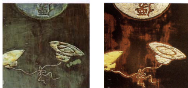
Figure 7. Black oil paint that had penetrated under the surface (a) was removed, revealing the earliest repair (b) made with traditional materials.
