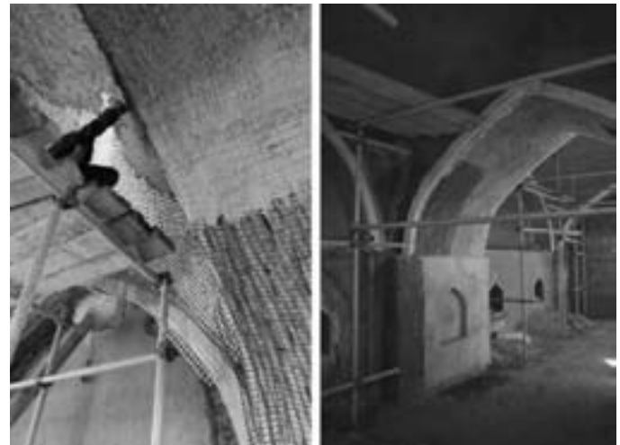
FIGURE 4 Reinforcement of the internal surfaces of the dome and walls in the Stable of the Citadel with geo-grids.
