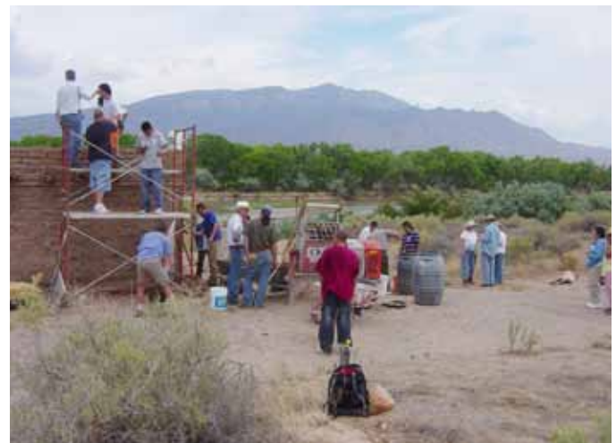
FIGURE 4 Work on a small building at the Coronado State Monument and the application of mud plaster. Photo: Francisco Uviña, 2006
