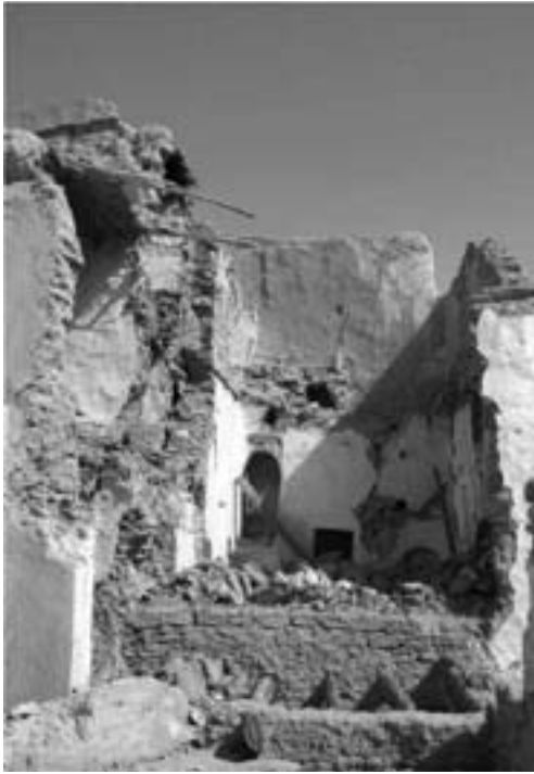
FIGURE 2 Deterioration of adobe structures in Ghadames. Photo: A Abufayed
