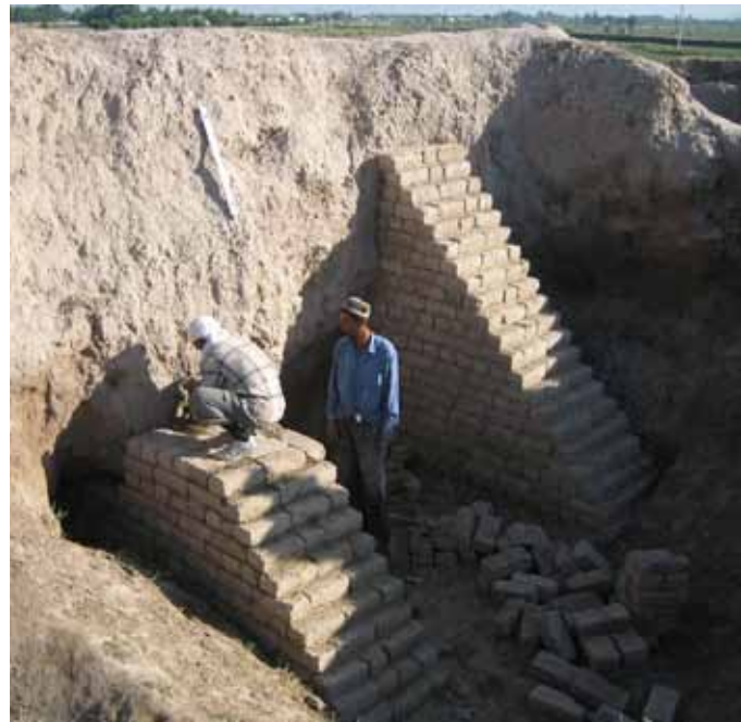
FIGURE 7 Construction of buttresses for the consolidation of leaning walls. Spring 2007. Photo: Enrico Fodde
