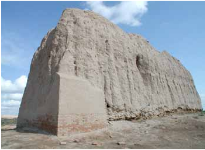
FIGURE 2 Kepter Kana in Merv, Turkmenistan. Corner repair using the traditional building technique of fired bricks at the wall base. Photo: Gaetano Palumbo. © World Monuments Fund
