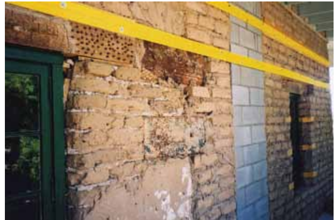
FIGURE 5 Polyester strapping in place at Los Luceros Hacienda, Alcalde, New Mexico. Photo: Edward Crocker
