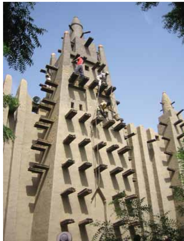
FIGURE 6 The first yearly crépissage in the Mopti mosque following restoration of the building in 2006. Periodic maintenance is of paramount importance for extending the life of earthen structures. Photo: AKTC, G. Taxil
