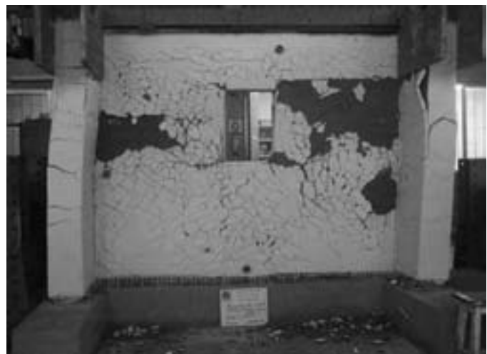
FIGURE 5 Wall with reinforcement of geo-grid and plastered with mud stucco. After cyclic shear test.
