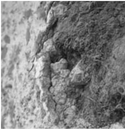
FIGURE 5 Cottown Schoolhouse: the lime base coat has lost coherence, while the topcoat and limewash remain sound.
