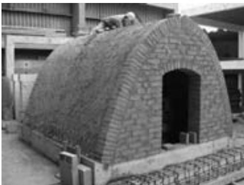
FIGURE 3 Nubian vault, without reinforcement of geo-grid and without mud stucco. Photo: Daniel Torrealva
