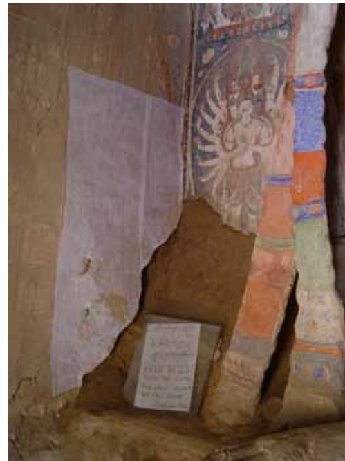
FIGURE 3 Erosion at the base of the wall. Photo: Bhawna Dandona
