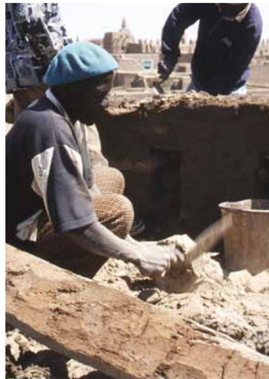
FIGURE 3 Masons and apprentices constructing the monumental parapet of a Djenné house. Photo by T. H. J. Marchand
