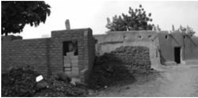
FIGURE 4 New and old buildings in Daura. Note the use of cellular concrete bricks for aeration purposes to the top left of the building under construction. Photo: Ishanlosen Odiava
