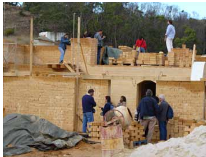
FIGURE 2 CEB construction in Carrapateira, Algarve. Visit during the IV SIACOT, held in Monsaraz, Portugal, in October 2005. Photo: Mariana Correia
