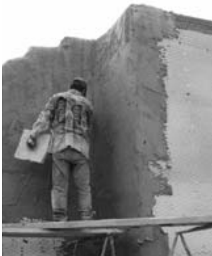
FIGURE 2 The application of cementitious plaster over wire lathe in Santa Fe, New Mexico, showing the lack of use of traditional plasters. Photo: Luis Fernando Guerrero Baca, 2006
