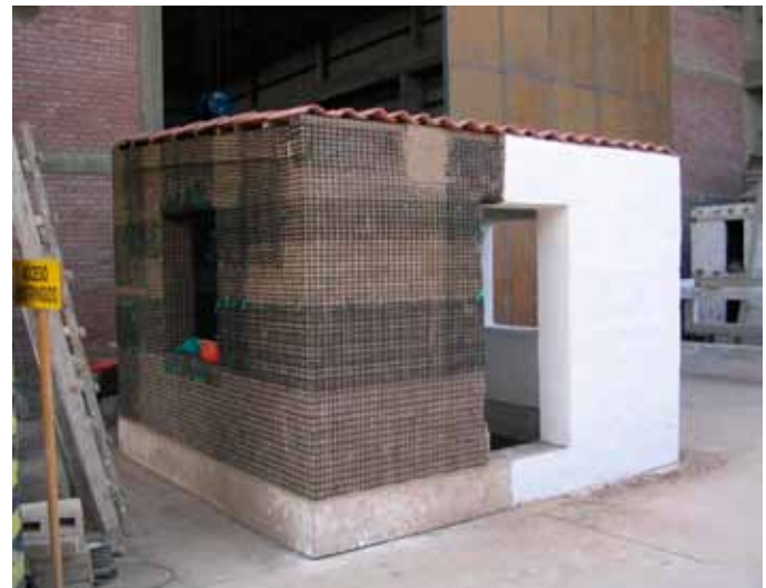
FIGURE 2 Square house reinforced with geo-grid, with mud plastered on one half of the module and not on the other half. Photo: Daniel Torrealva
