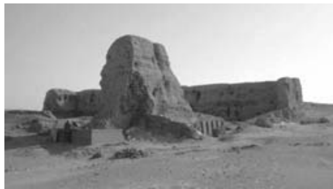
FIGURE 5 View of the northeast corner, which collapsed in 2002, and ongoing repairs in 2007. Photo: R. Jaeschke
