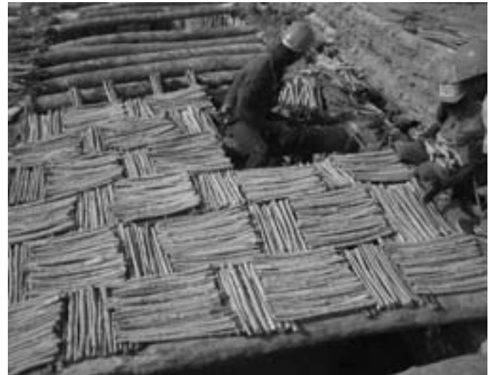
FIGURE 4 Installation of the ceiling made of goettes arranged in a geometric pattern, part of the work on the roof of the Djingareyber mosque. Photo: AKTC, M. Sy
