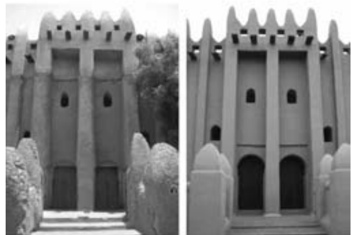
FIGURE 2 The south entrance of the Mopti mosque before and after restoration. Note the damage caused by the cement structure constructed on top of the building prior to restoration of the structure. Photos: AKTC, G. Devreux and G. Taxil
