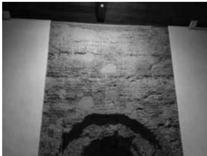
FIGURE 5 Detail of the top of a rammed earth wall after treatment with saliva de cupim. Photo: © Honório Nicholls Pereira
