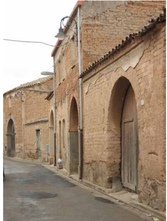
FIGURE 4 Adobe buildings along a road in Serramanna. Photo: Department of Architecture, Faculty of Architecture of Cagliari.
