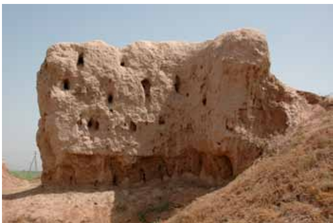
FIGURE 5 One of the tallest earthen walls after removal of vegetation showing decay caused by bird nesting. Spring 2006. Photo: Enrico Fodde
