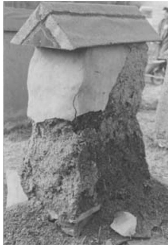
FIGURE 4 ESRP cement-rendered wall: showing major damage that subsequently led to collapse of the wall.
