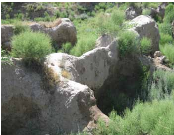
FIGURE 4 Vegetation is one of the main deterioration factors for the earthen walls of Ajina Tapa. Deep roots (up to 1.5 m) expand while growing and cause collapse of parts of the wall. Spring 2006. Photo: Enrico Fodde
