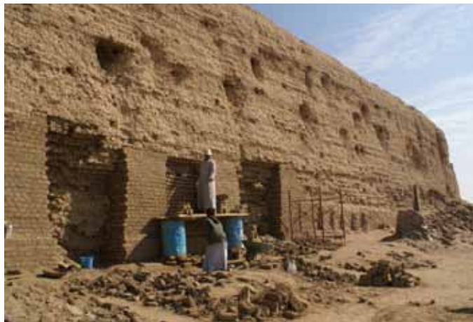
FIGURE 6 Repair of the exterior west wall with a series of buttresslike constructions that were later interbonded. Photo: R. Friedman
