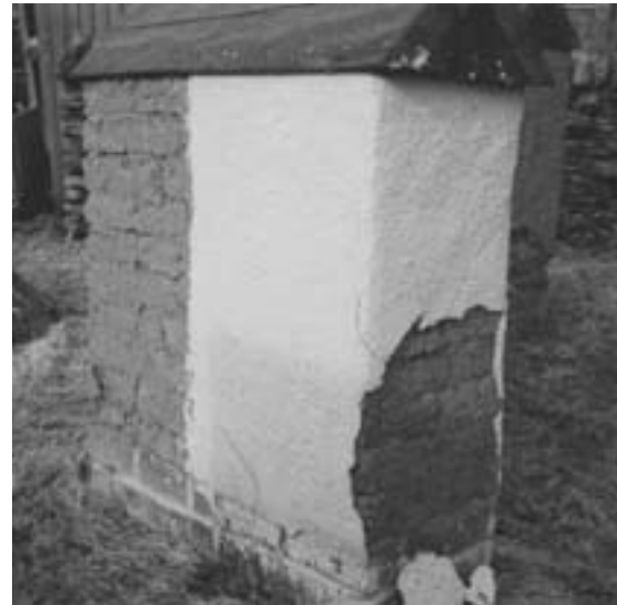
FIGURE 3 ESRP lime-rendered wall: showing loss of bond but not damage to the earth wall.
