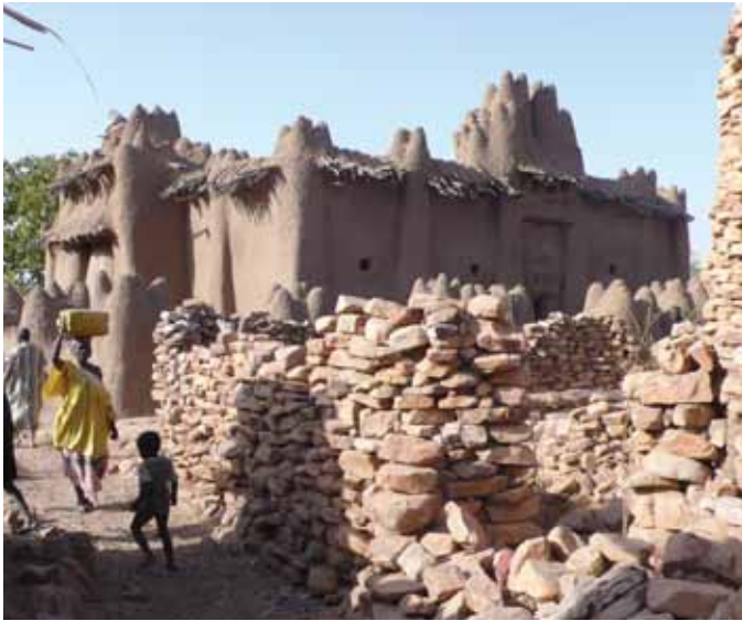
FIGURE 5 The mosque of Nando, in a small village near Mopti, is one of many traditional earthen structures that need to be inventoried, listed, and protected. Photo: AKTC, G. Taxil
