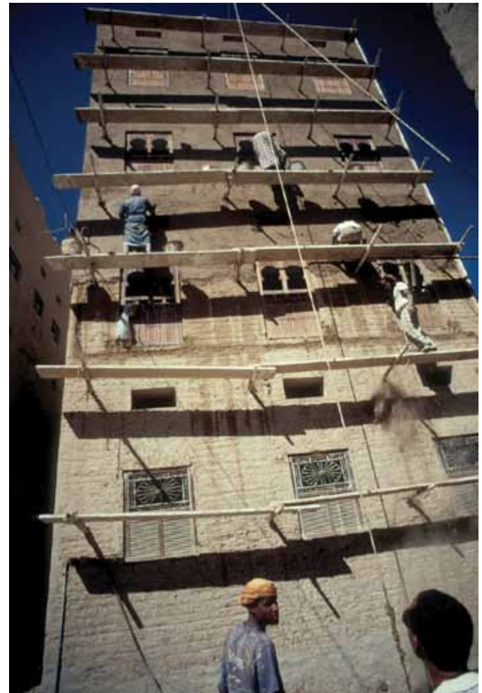
FIGURE 4 Traditional builders applying a coat of mud plaster. Photo: Pamela Jerome. Courtesy of the Visual Media Center, Columbia University
