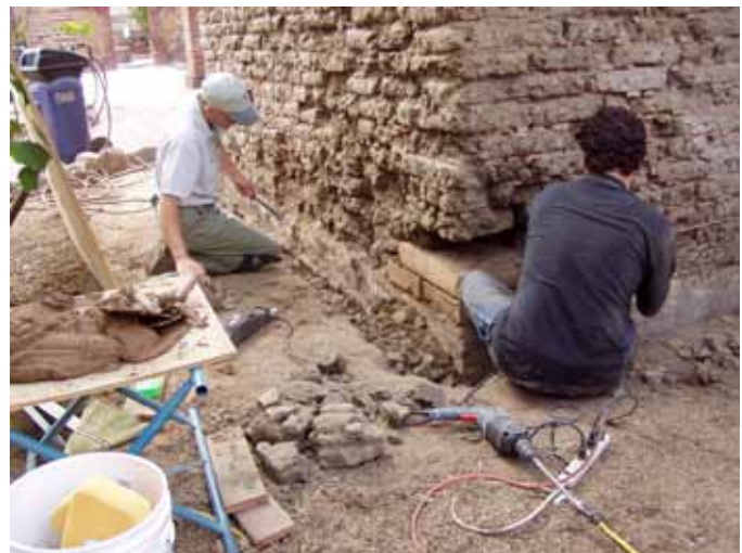
FIGURE 4 Maintenance of the base of adobe walls is critical to their seismic performance.
