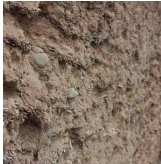
FIGURE 6 Moorhouse Washhouse: removal of cement render revealed a coarse mud wall with lines of straw layers.
