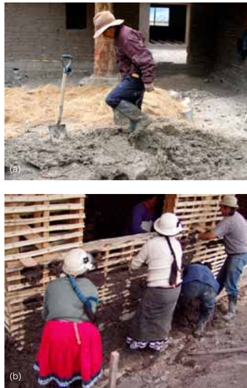
FIGURE 3 The Cañar House, constructed of wattle-and-daub, a mixture of mud and straw packed into a wooden latticework. Photos: Lourdes Abad R., 2006
