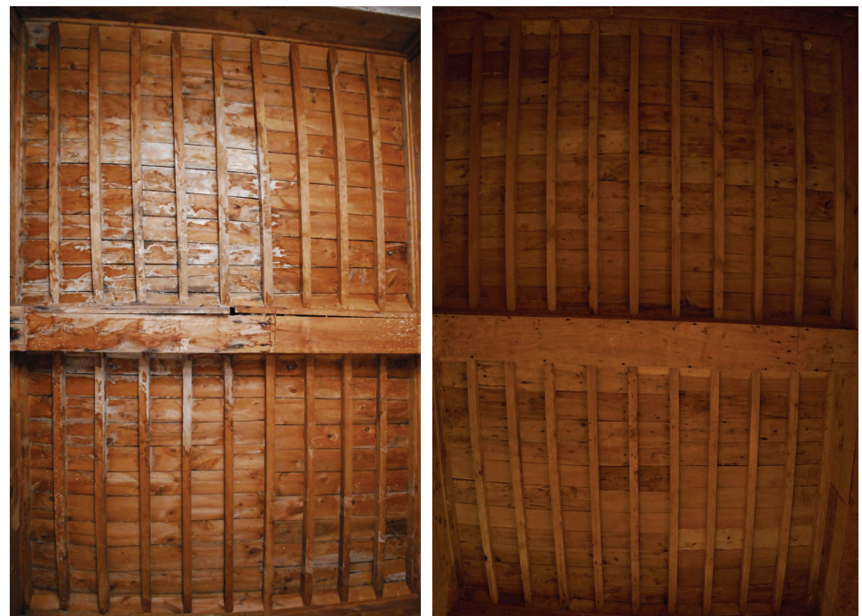
FIGURE K.27A AND K.27B Wood ceiling, Stara East before (left) and after (right) implementation.
