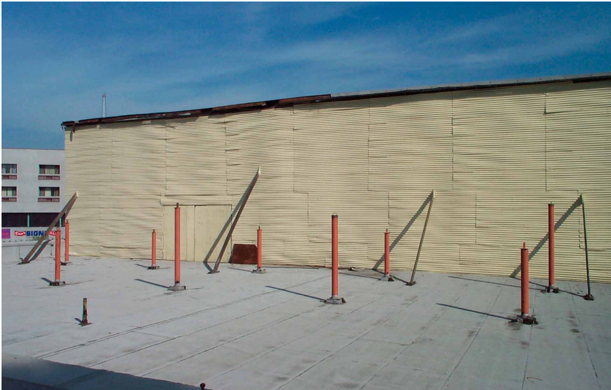
Figure 1 One of a series of protective coverings erected over the mural since 1982. The steel columns in the foreground were intended to support a future mural shelter. Photo: Brooks + Scarpa
