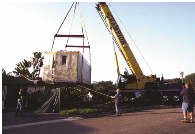
Figure 5 Ted Hollinger of Master House Movers and his crane operators, on site in Pacific Palisades, lifting the twenty-five-ton mural-building onto a lowboy tractor-trailer headed for Santa Barbara. Photo: Siqueiros Mural Project Team, Courtesy Santa Barbara Museum of Art
