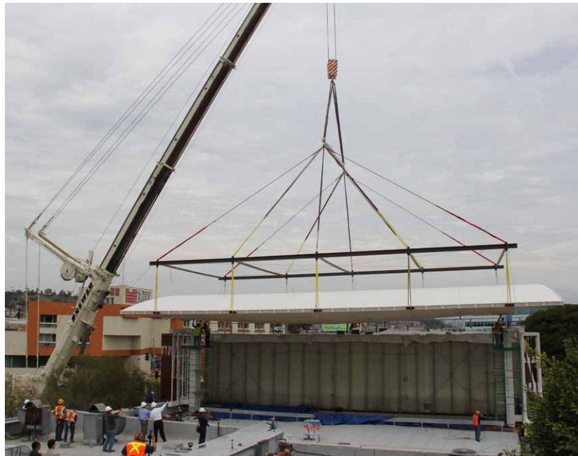
Figure 10 The crane positioning the canopy on top of the columns above the roof of the Hammel Building. Photo: City of Los Angeles; mural: © 2012, Artists Rights Society (ARS), New York/Sociedad Mexicana de Autores de las Artes Plásticas (SOMAAP), Mexico City
