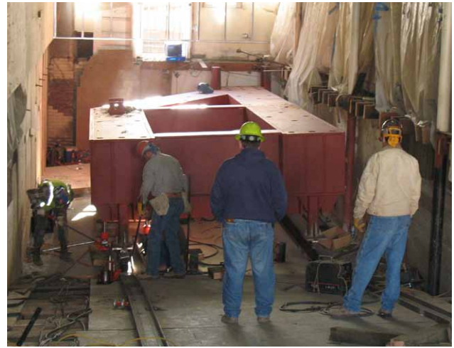
Figure 6 The transfer beam in its final position. Photo: City of Los Angeles
