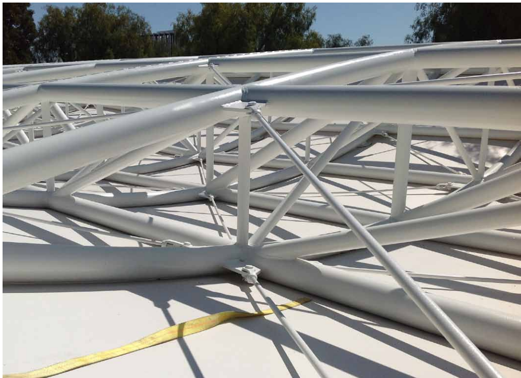
Figure 7 The installation of the fabric on the canopy structure, done in a parking lot across the street from the mural. Photo: City of Los Angeles
