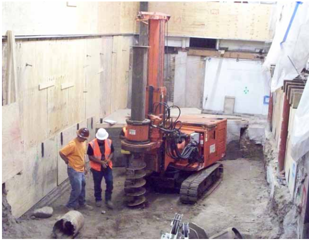
Figure 5 Pile drilling in a confined space inside the Hammel Building. Photo: City of Los Angeles
