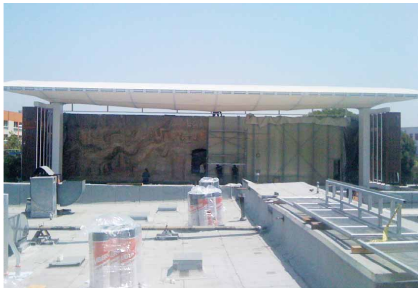
Figure 11 The canopy after installation. Photo: City of Los Angeles; mural: © 2012, Artists Rights Society (ARS), New York/Sociedad Mexicana de Autores de las Artes Plásticas (SOMAAP), Mexico City
