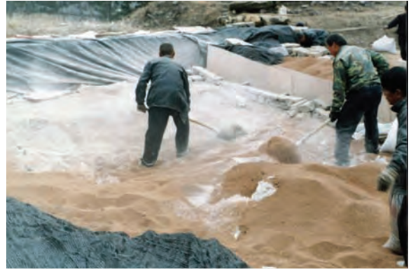
2. 清凉楼，混合回填用的黄土与石灰 Qingliang Building, reburial, mixing soil with lime
