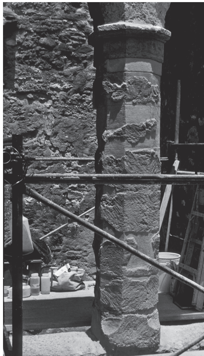
FIGURE 7 Convent of Mission San Jose, San Antonio, Texas. Stone consolidation and mortar repairs were identified as the most minimal interventions necessary to stabilize and reinstate the form but preserve the original fabric of this unique column on site. Photo: Frank Matero
