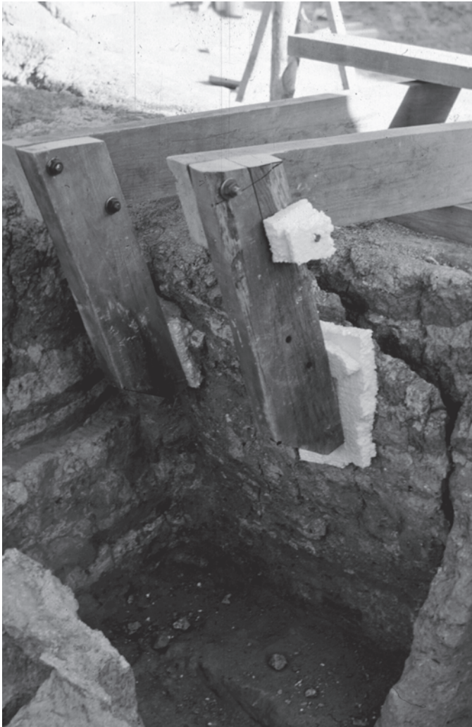
FIGURE 2 Çatalhöyük, Turkey. Structural collapse and plaster surface delamination occur almost immediately on exposure and require both large- and small-scale temporary treatments during and after excavation. Photo: Frank Matero
