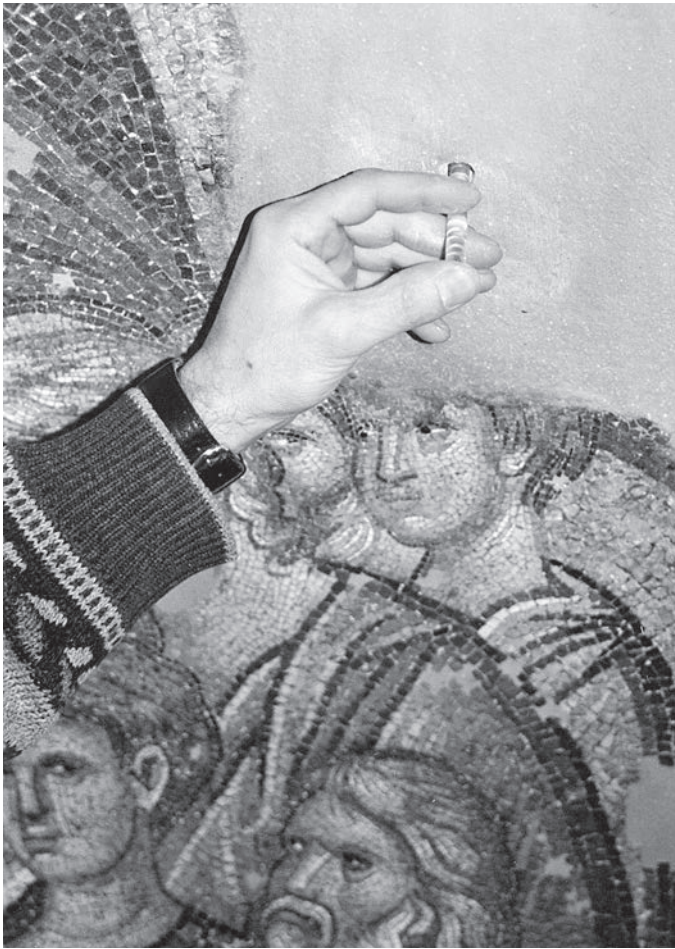
FIGURE 4 Stabilization of the mortar bedding on the masonry with Plexiglas anchor rivets. Photo by C. Bakirtzis.
