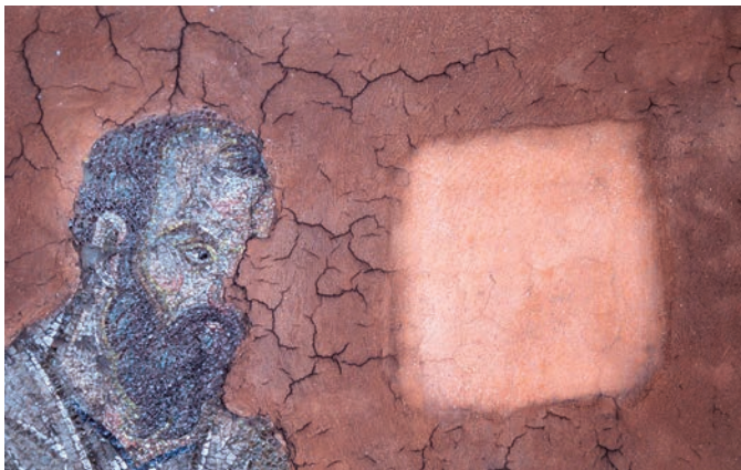
FIGURE 7 Trial cleaning of the neutral plaster (dome, prophet Isaiah). Photo by C. Bakirtzis.
