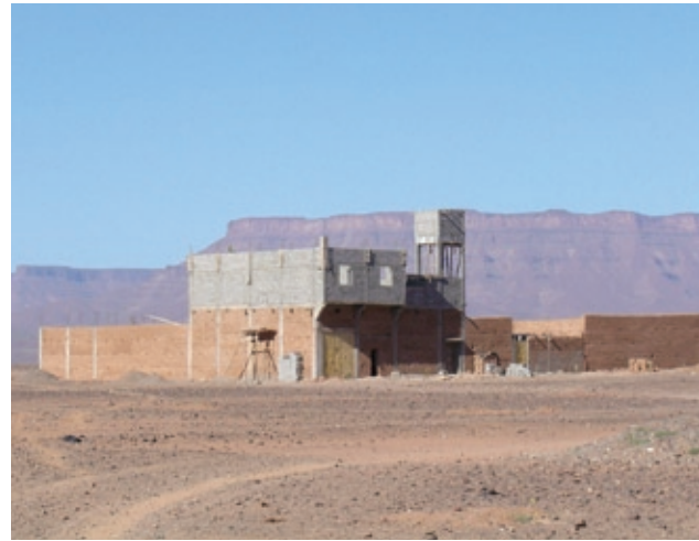
FIGURE 11 Structure exhibiting a mix of materials that reveals ignorance of rules of good practice.
