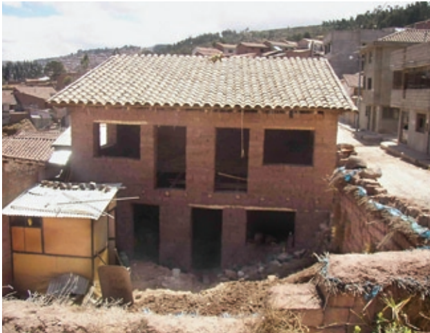
FIGURE 1 Seismically vulnerable adobe house in Peru.
