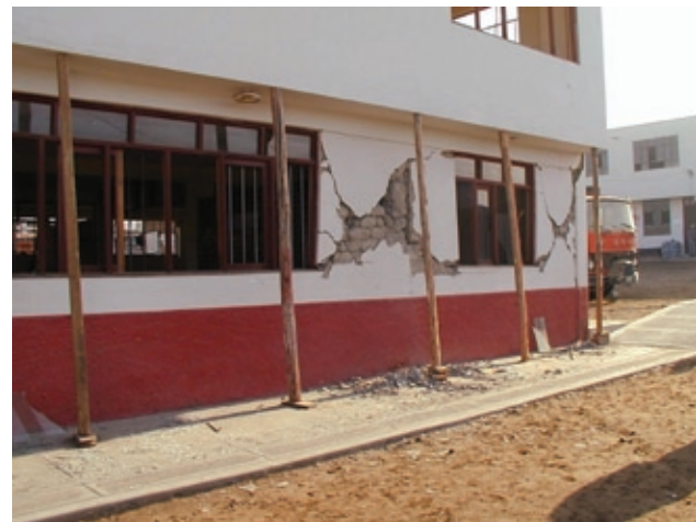
FIGURE 2 Seismic cracks of unreinforced adobe house.
