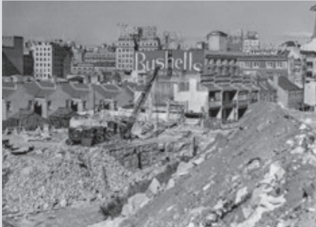
FIGURE 6 Excavation through The Rocks for construction of the Cahill Expressway's southern approach to the Sydney Harbour Bridge in 1955.
