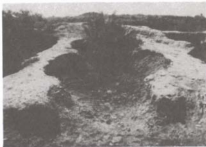
Figure 10. A view of the "Archives" in Seleucia. The top of the walls was capped with soil-cement, which did not prove to be effective, since there was formation of water pools at the bases of the walls.
