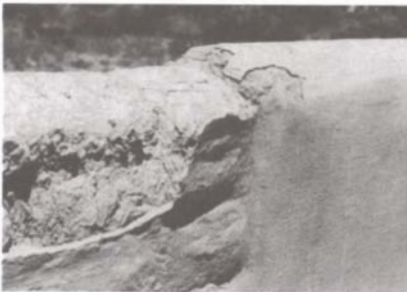
Fig. 8 Detail of the erosional pattern on the Super Quickseal panel.
