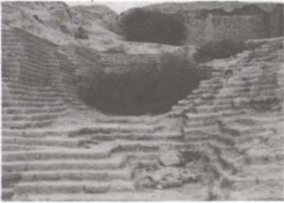
Figure 8. The canalization of rain water over Tell 'Umar. In spite of some plant growth and some minor damage, this drainage system worked properly.
