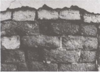
Figure 15. Wall treated with ethyl silicate in Hatra, as it appeared in 1969. The top layer of bricks was not consolidated.
