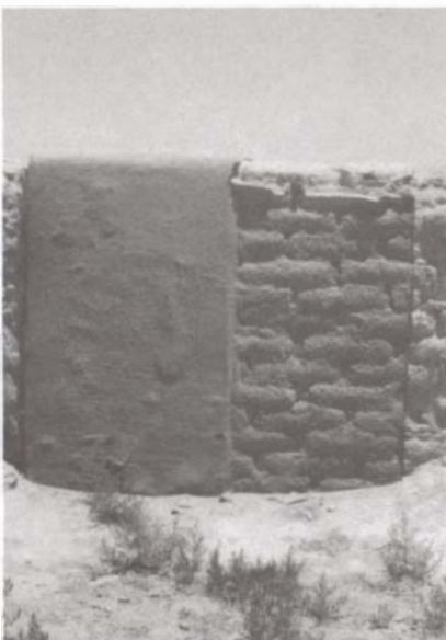
Fig. 9 Thorocoat panel. Note cracks and deteriorating coating.
