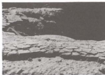
Figure 12. Detail of the soil-cement capping, partially detached and cracked. Besides damage due to temperature changes and water infiltration, it should be remembered that people walked on the capping.
