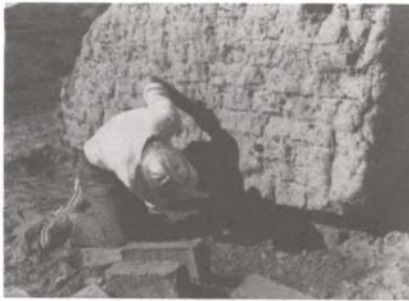
Workman preparing eroded wall base for insertion of new adobe bricks, 1974. New Mexico State Monuments.
