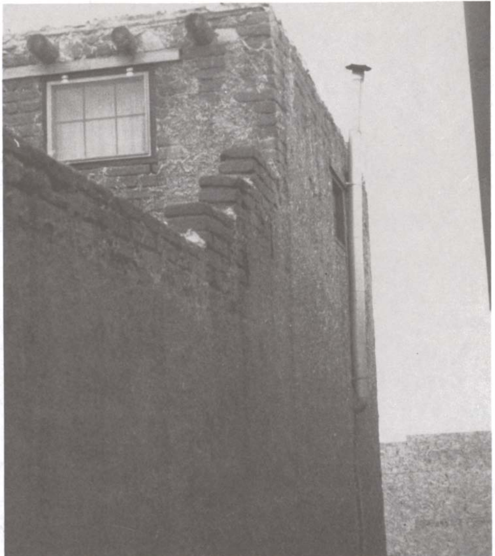
Mud plaster erosion from asphalt stabilized adobe bricks.
