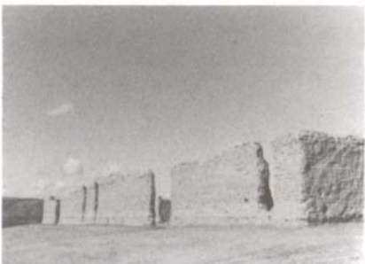
Adobe wall after stabilization, 1974. The ground surface has been raised to provide wall support and graded to facilitate water runoff. New Mexico State Monuments.
