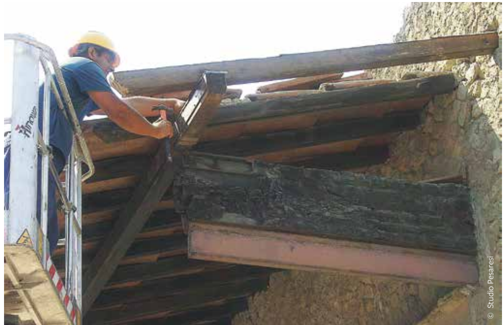
FIGURE 13: Maintenance of a shelter in Herculaneum, Italy (see the chapter by Pesaresi and Massari in this publication).
