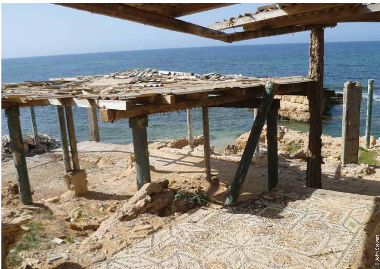
FIGURE 8: The Villa of the Nereids, Tajurah, Libya, with its steel and wooden shelter erected after excavation in the 1960s. After decades of neglect, the structures are in a dangerous state of collapse from corrosion of the metal supports.
