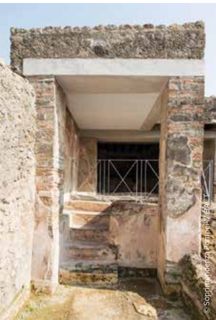
FIGURE 5: An example of a flat shelter in concrete at the Fullonica of Stephanus.
