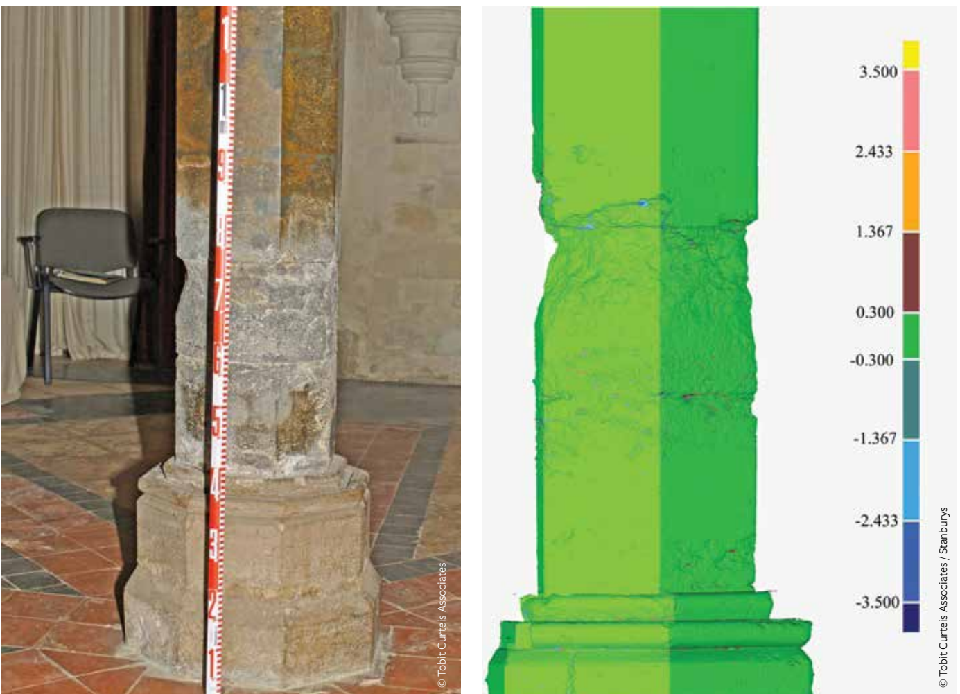
FIGURE 4: Periodic laser scanning was used to evaluate minor condition changes in the medieval columns at Anglesey Abbey, UK.
