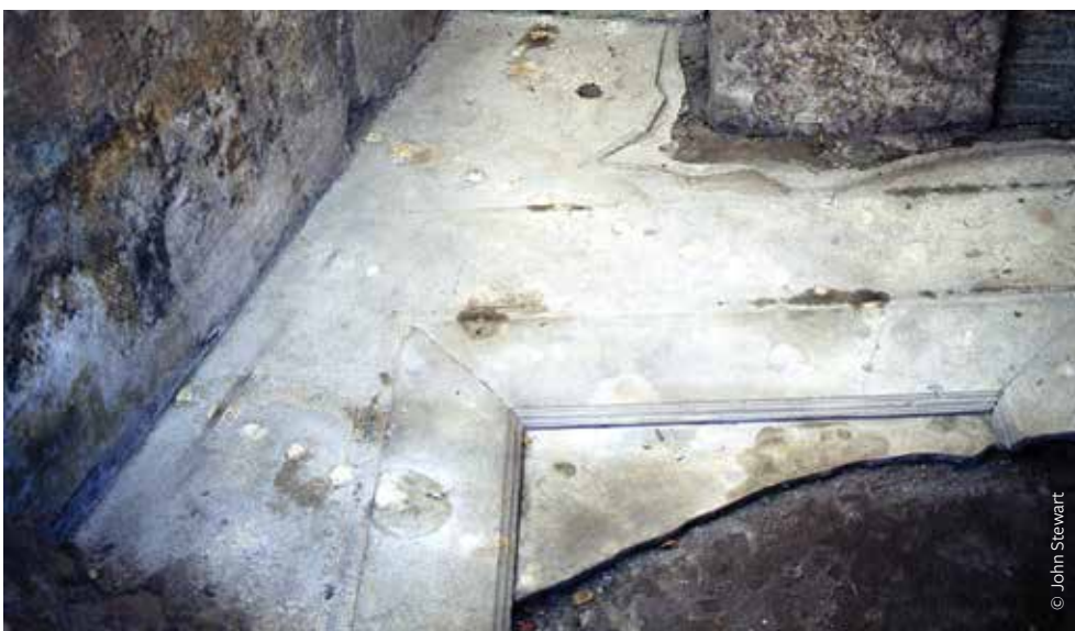
FIGURE 7: Water droplets on a marble floor, from holes in the shelter roof caused by corrosion of metal fasteners.
