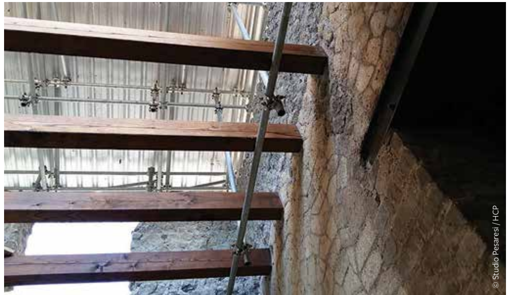
FIGURE 24: In Herculaneum a provisional shelter is secured to wooden joists that will eventually support a permanent flat roof. This ensures immediate protection. In addition, since specific beams are supporting the weight of the temporary roof, the scaffolding props can be moved or removed as necessary to allow the space required to build the permanent roof over time (see the chapter by Pesaresi and Massari in this publication).
