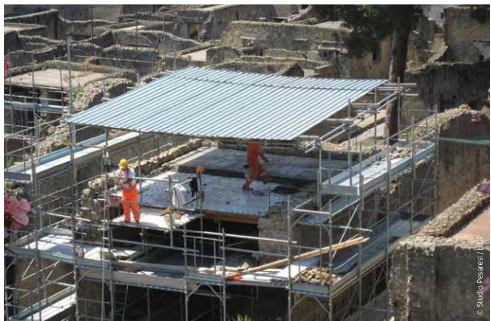
FIGURE 4: A site-wide conservation campaign saw repairs take place on modern shelters throughout Herculaneum. Where the original Roman structure does not survive up to its roof height the original floor slab of an upper floor in the building has often been used as the basis of a new covering.
