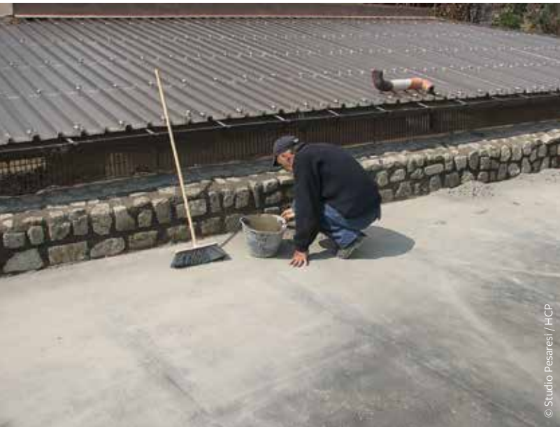
FIGURE 17: An example of preventive maintenance on a floor slab that serves as a shelter for the room below in Herculaneum: this includes removing dust and vegetation, and sealing gaps between the external wall and the waterproof layer (see the chapter by Pesaresi and Massari in this publication).
